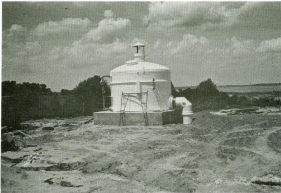
Activated Carbon Air Filter For The Wet Well
