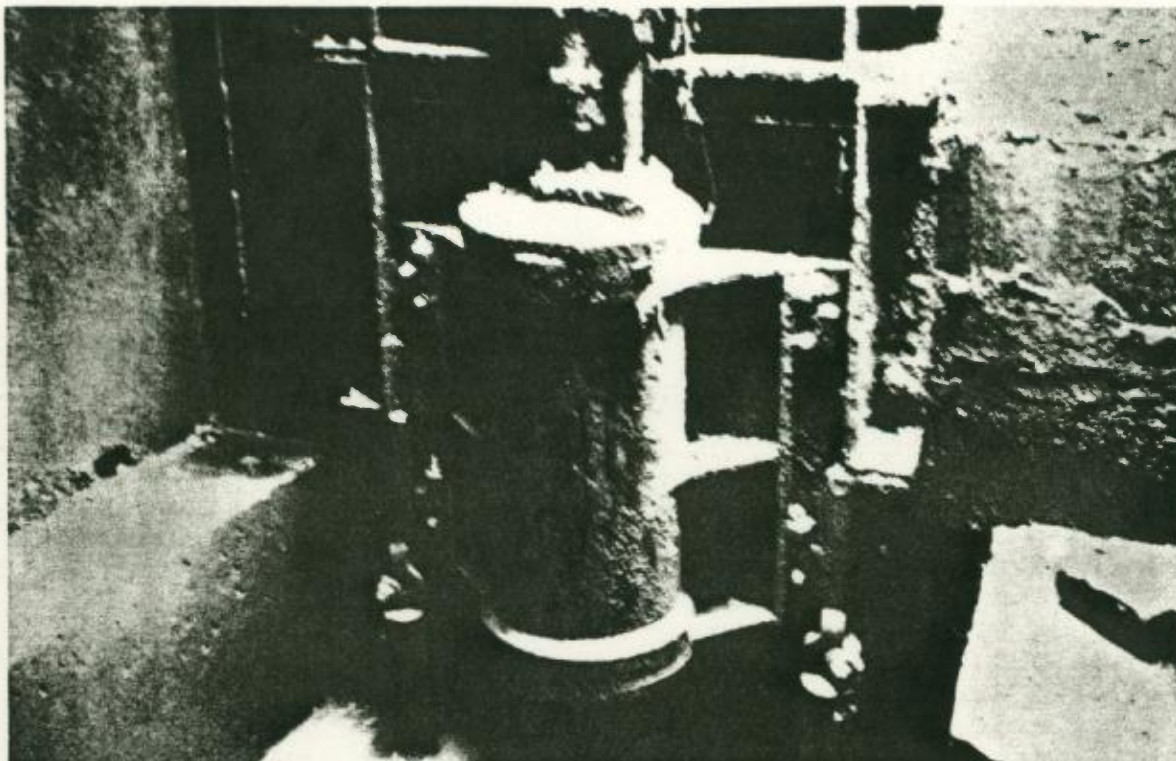
FIG. 10-A, HYDRAULICALLY OPERATED SLUICE GATE AT REGULATOR 6 (CONTRACT 2), NICHOLAS AVENUE AND RICHMOND TERRACE, PORT RICHMOND, NEW YORK
