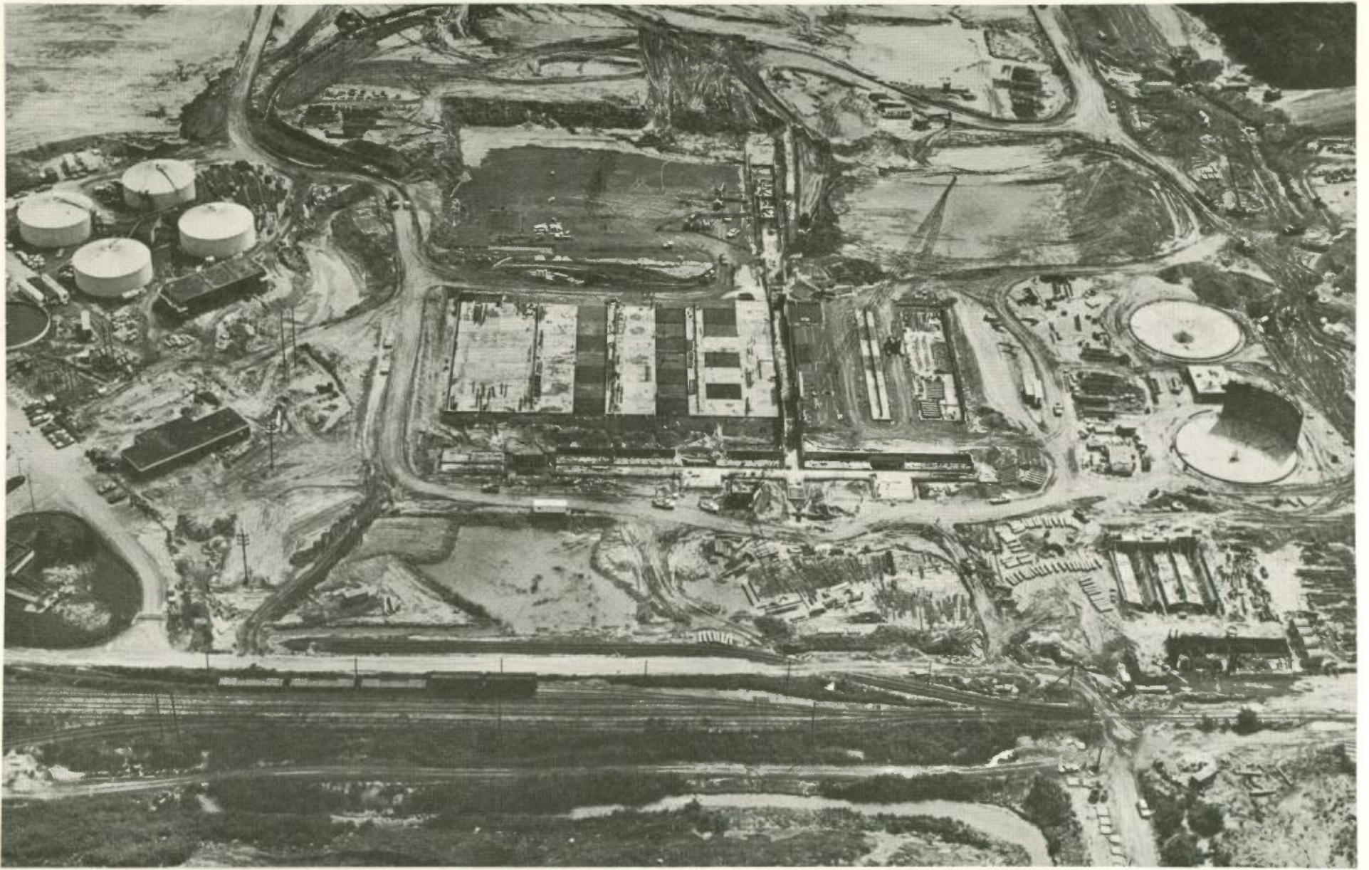
CONSTRUCTION AT THE MIDDLESEX COUNTY SEWERAGE AUTHORITY TREATMENT PLANT, MIDDLESEX COUNTY, N.J. Consulting Engineers: Metcalf and Eddy, Inc.
